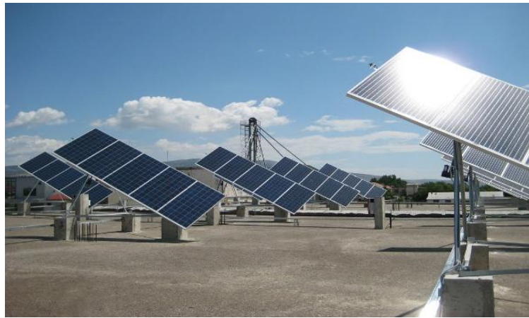
Trikala1: 19.80 kWp single axis
