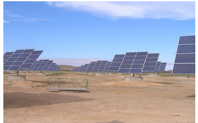
Valdespino Park 4: 106,92 kWp
