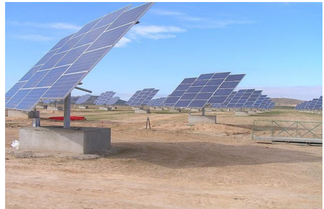
Valdespino Park 3: 106,92 kWp
