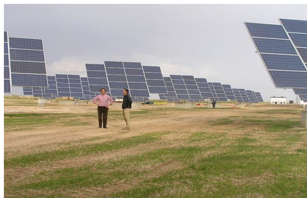
Valdespino Park 5: 106,92 kWp
